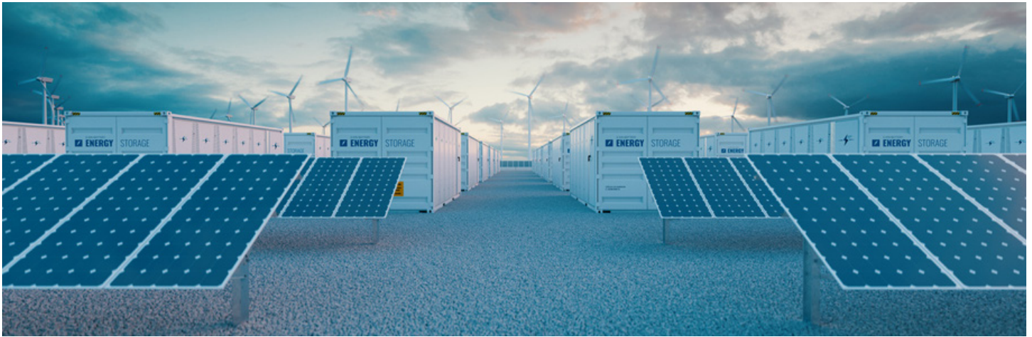
Large-scale BESS installations supporting grid stability and power demand
